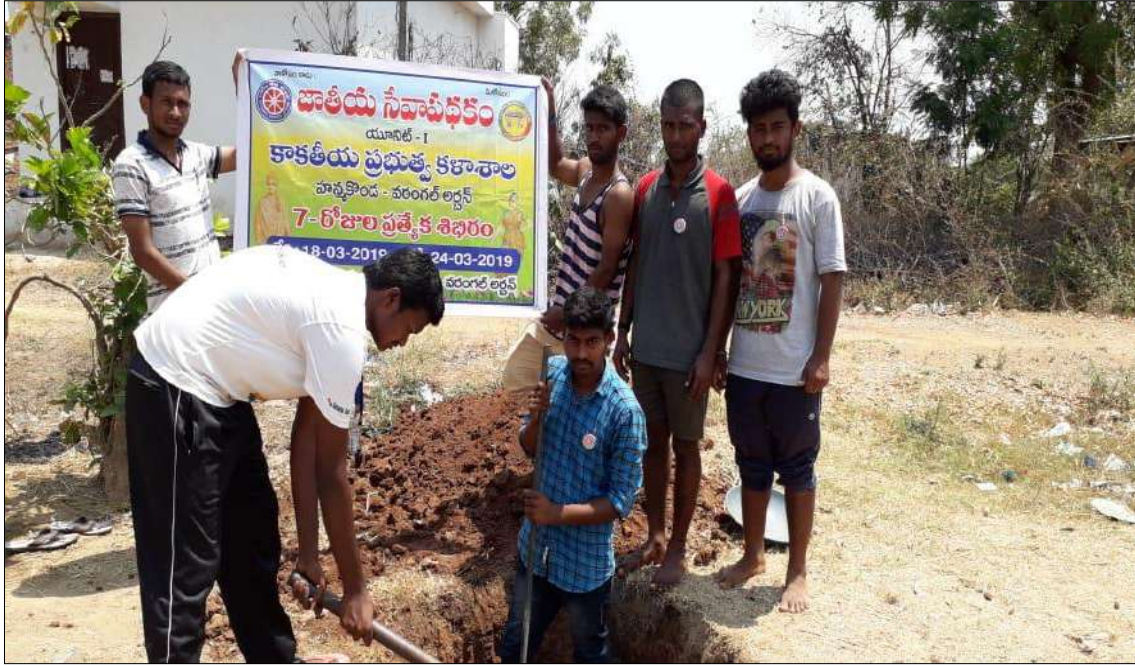
As a part of Special camp, The NSS volunteers digging the Latrine pits for the villagers on 22-03-2019
